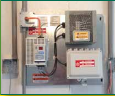
VFD Controls for variable speed operation
